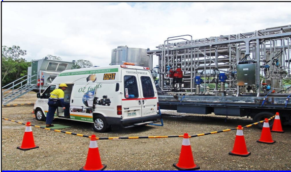
Oz Future Fuels on-site hydrocarbon recycling plant
