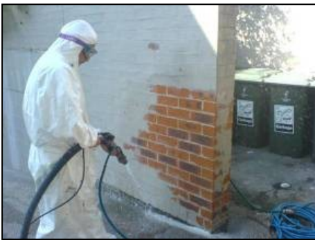
Photo: Sodablasting has many ‘in-demand’ applications. Photo shows an operator removing stubborn paint layers from masonry without damage to mortar.
