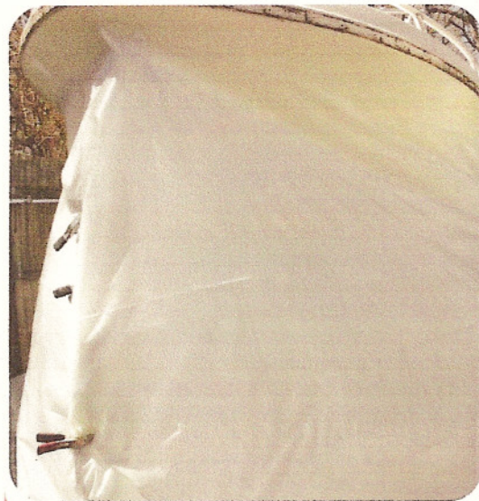
IT'S A WRAP: The hull is totally sealed off from the environment.
