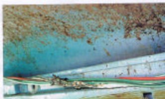
Burnt out wiring and grape vine remains.
